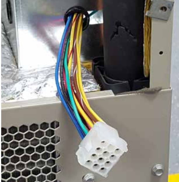
FIGURE 9 Low Voltage Wire Harness Pulled Through Grommet
