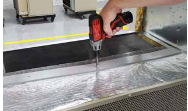
FIGURE 4 New Condenser Exhaust Plate with Screen
