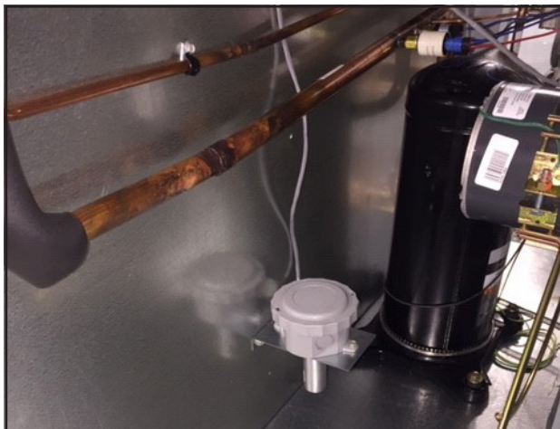
FIGURE 18 Temperature Only Sensor Assembly Installation
