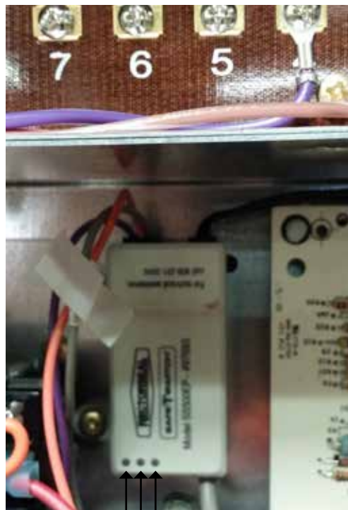
FIGURE 32 Outdoor Condensate Control
