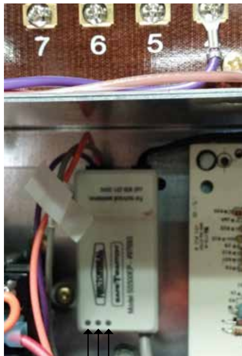
FIGURE 32 Outdoor Condensate Control
