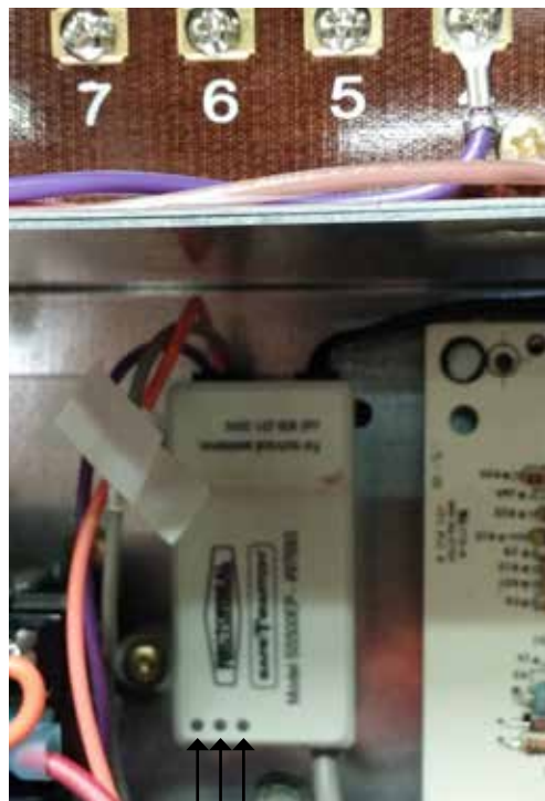
FIGURE 36 Outdoor Condensate Control
