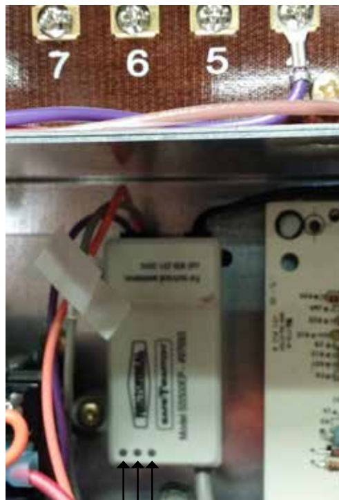
FIGURE 36 Outdoor Condensate Control
