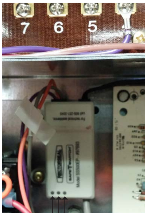
FIGURE 36 Outdoor Condensate Control
