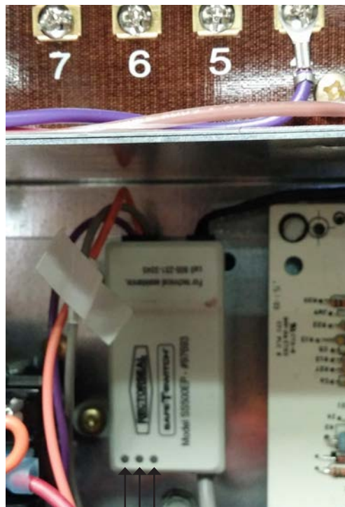
FIGURE 36 Outdoor Condensate Control
