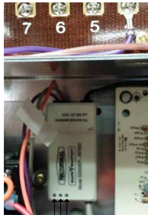
FIGURE 20 Outdoor Condensate Control
