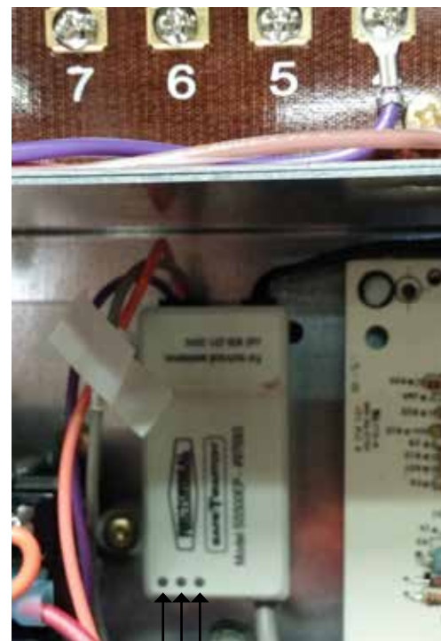
FIGURE 20 Outdoor Condensate Control
