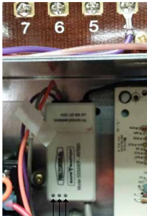
FIGURE 28 OUTDOOR CONDENSATE CONTROL
