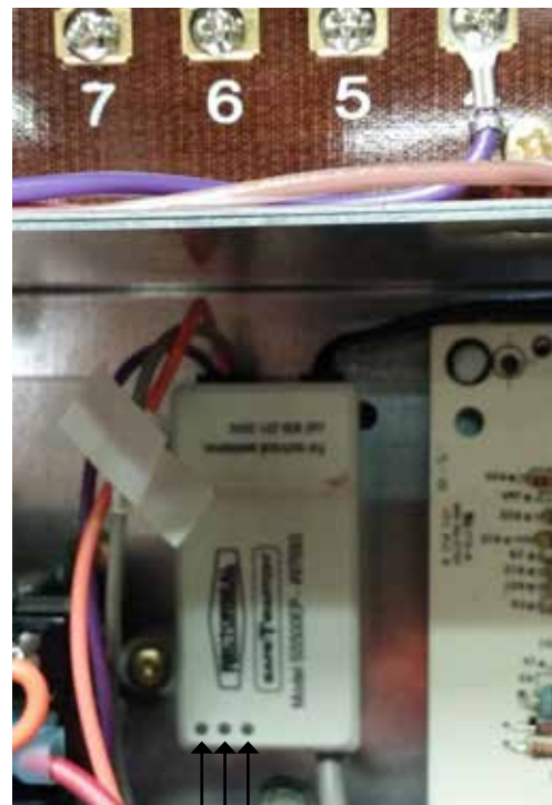
FIGURE 35 Outdoor Condensate Control
