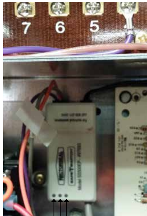
FIGURE 35 Outdoor Condensate Control
