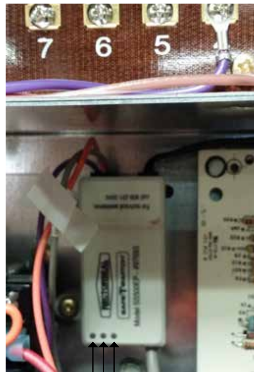
FIGURE 35 Outdoor Condensate Control
