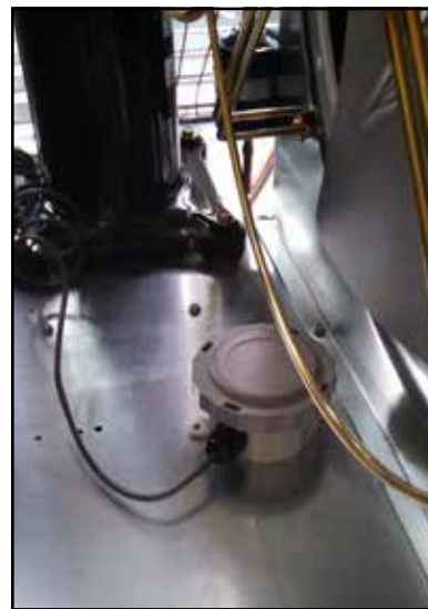
FIGURE 1.3 Outdoor Sensor Installation
