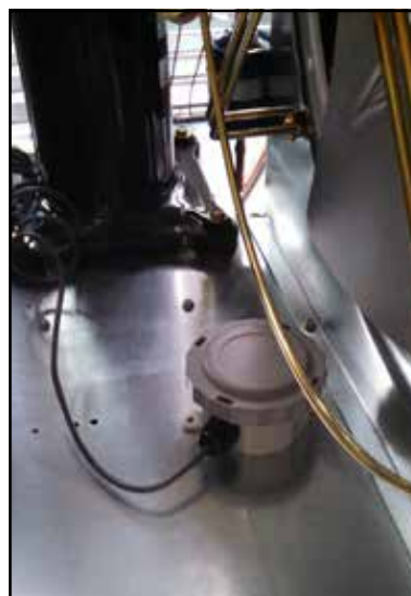
FIGURE 1.3 Outdoor Sensor Installation
