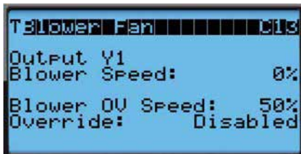
FIGURE 15 Putting Blower Output into Override Mode
