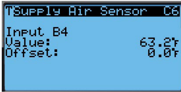
FIGURE 37 Supply Air Sensor
