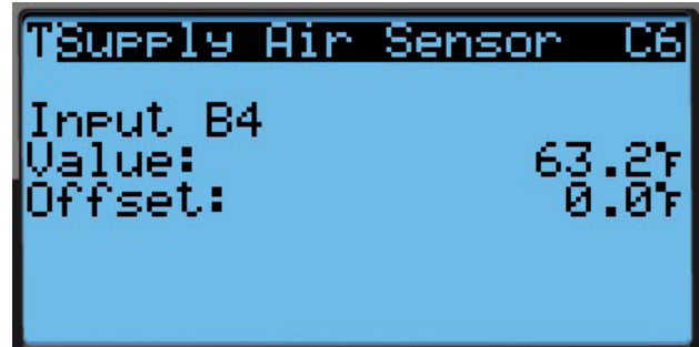
FIGURE 39 Supply Air Sensor
