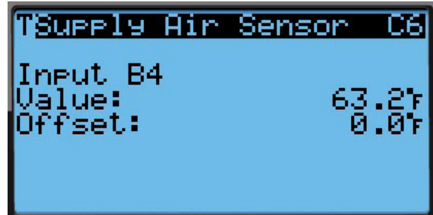
FIGURE 39 Supply Air Sensor
