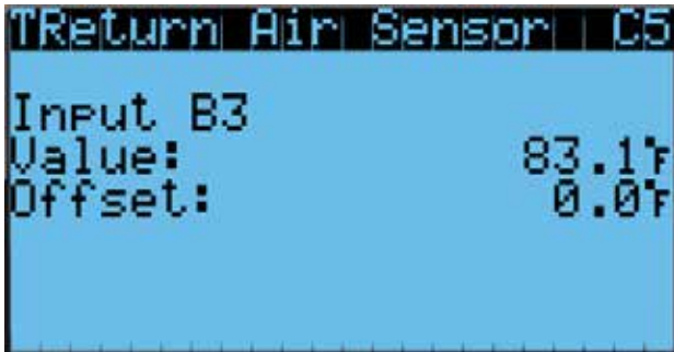
FIGURE 20 Adjusting Return Air Sensor
