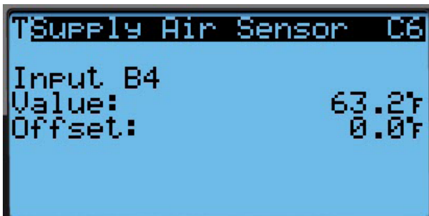
FIGURE 53 Supply Air Sensor
