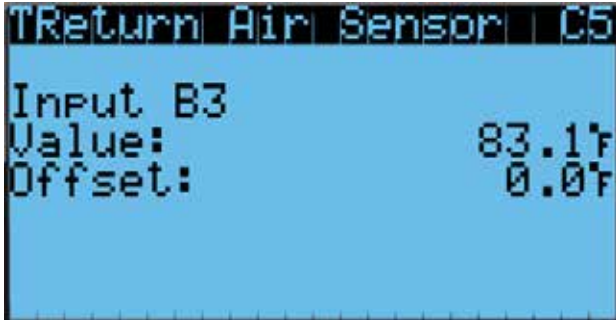
FIGURE 20 Adjusting Return Air Sensor
