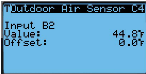
FIGURE 49 Outdoor Air Sensor
