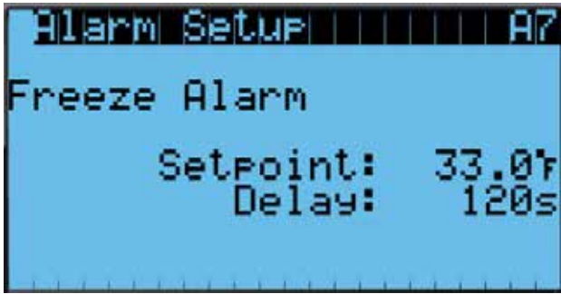
FIGURE 28 Adjusting Freeze Setpoint and Alarm Delay
