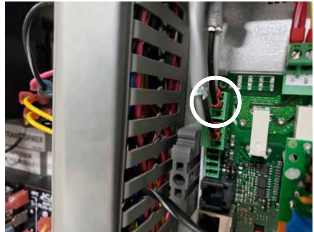
FIGURE 62 Verify Modbus is Connected to PLC Board
