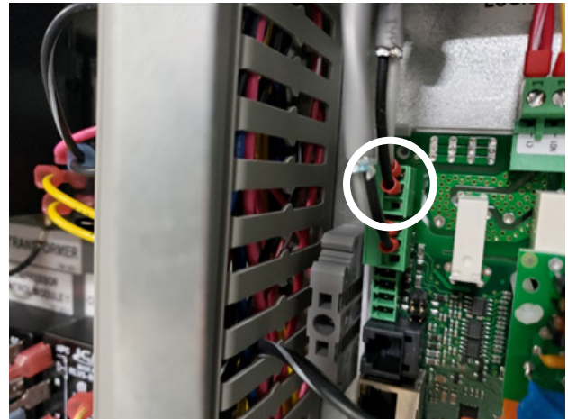
FIGURE 89 Verify Modbus is Connected to PLC Board
