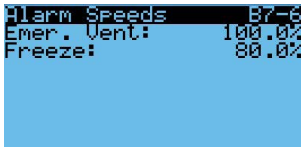
FIGURE 29 Adjusting Emergency Vent and Freeze Speeds
