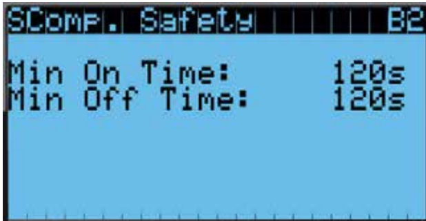
FIGURE 31 Adjusting Compressor Delays
