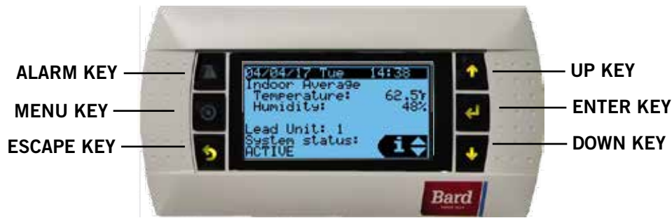
FIGURE 39 LV1000 Controller Display and Interface (Status Screen Shown)
