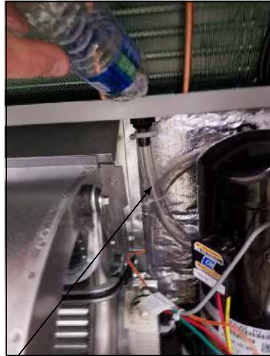
Evaporator Drain Pan Right Side Drain Hose
