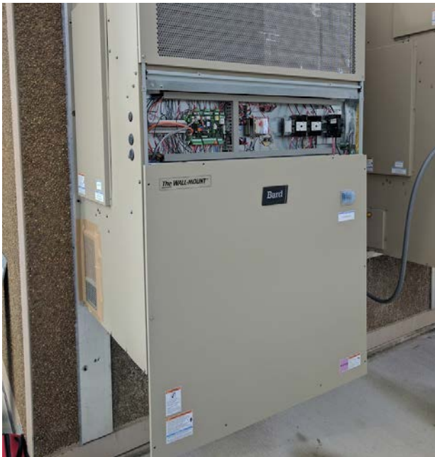
FIGURE 4 Hanging Front Access Panel to Allow Access to Control Panel
