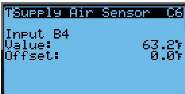
FIGURE 52 Supply Air Sensor
