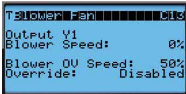
FIGURE 29 Putting Blower Output into Override Mode
