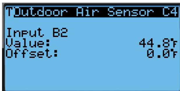
FIGURE 49 Outdoor Air Sensor
