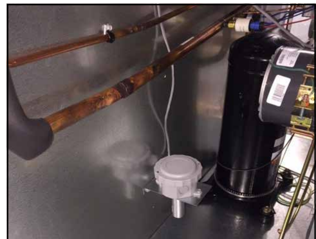
FIGURE 16 Temperature Only Sensor Assembly Installation
