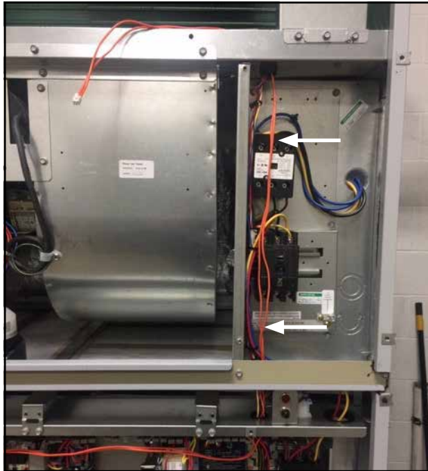
FIGURE 12 Route Orange Mixed Air Sensor Wires
