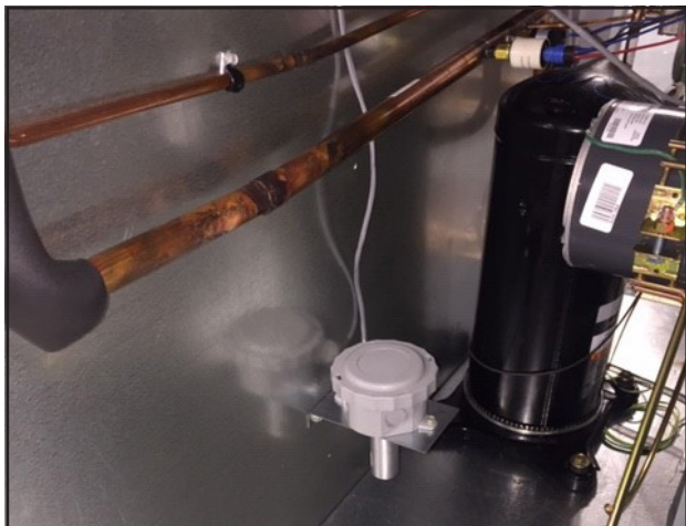
FIGURE 18 Temperature Only Sensor Assembly Installation
