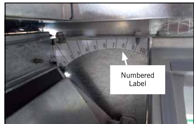
FIGURE 16 Ventilation Air Label
