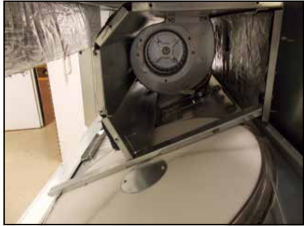
FIGURE 26 Upper Blower Assembly Over Cassettes
