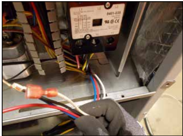
FIGURE 18 Feed Wires to Left Side of Unit
