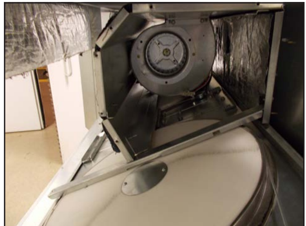
FIGURE 33 Upper Blower Assembly Over Cassettes
