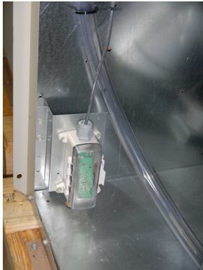
FIGURE 5 Outdoor Air Sensor Installation
