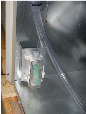
FIGURE 5 Outdoor Air Sensor Installation
