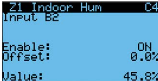
FIGURE 44 Enable/Disable Zone 1 Indoor Humidity Sensor
