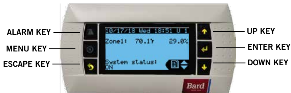
FIGURE 36 LC6000 Controller Display and Interface (Status Screen Shown)
