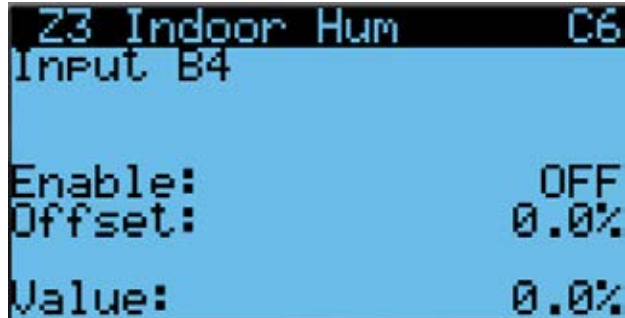
FIGURE 38 Enable/Disable Zone 3 Indoor Humidity Sensor
