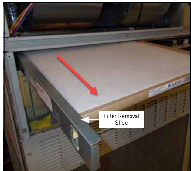
FIGURE 2 Removing Left Filter
