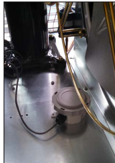
FIGURE 3 Outdoor Sensor Installation
