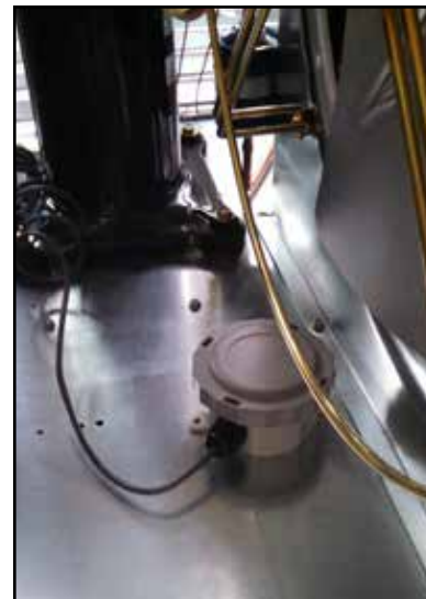
FIGURE 3 Outdoor Sensor Installation
