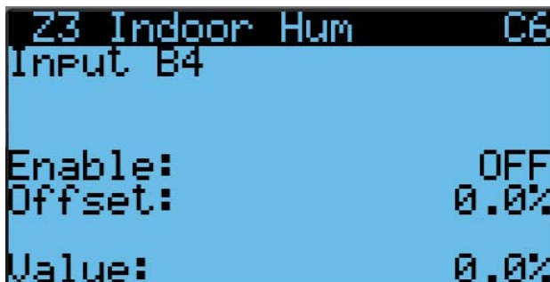
FIGURE 35 Enable/Disable Zone 3 Indoor Humidity Sensor
