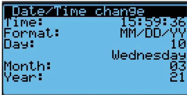
FIGURE 31 Setting Controller Date and Time
