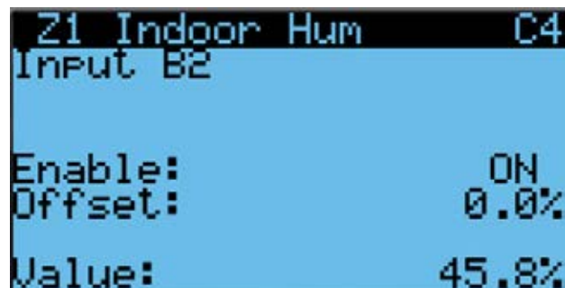
FIGURE 33 Enable/Disable Zone 1 Indoor Humidity Sensor
