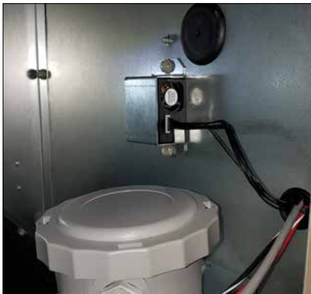
FIGURE 3 Dust Sensor Mounted on Partition Wall
