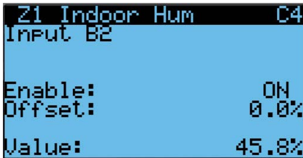
FIGURE 36 Enable/Disable Zone 1 Indoor Humidity Sensor
