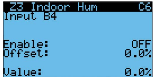
FIGURE 38 Enable/Disable Zone 3 Indoor Humidity Sensor
