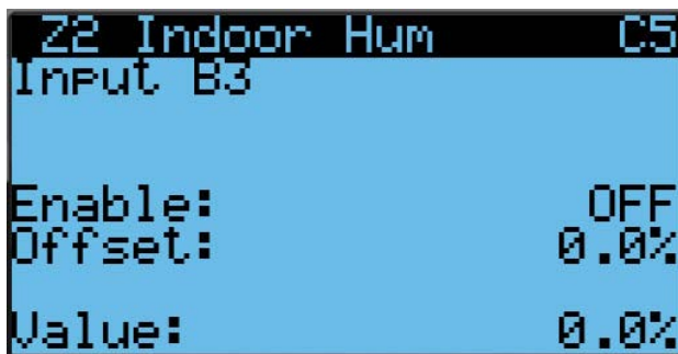
FIGURE 37 Enable/Disable Zone 2 Indoor Humidity Sensor
