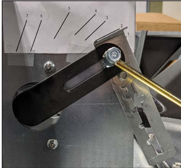
FIGURE 14 Set Blade Stop to Adjust Fresh Air Amount
