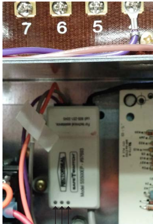
FIGURE 36 Outdoor Condensate Control
